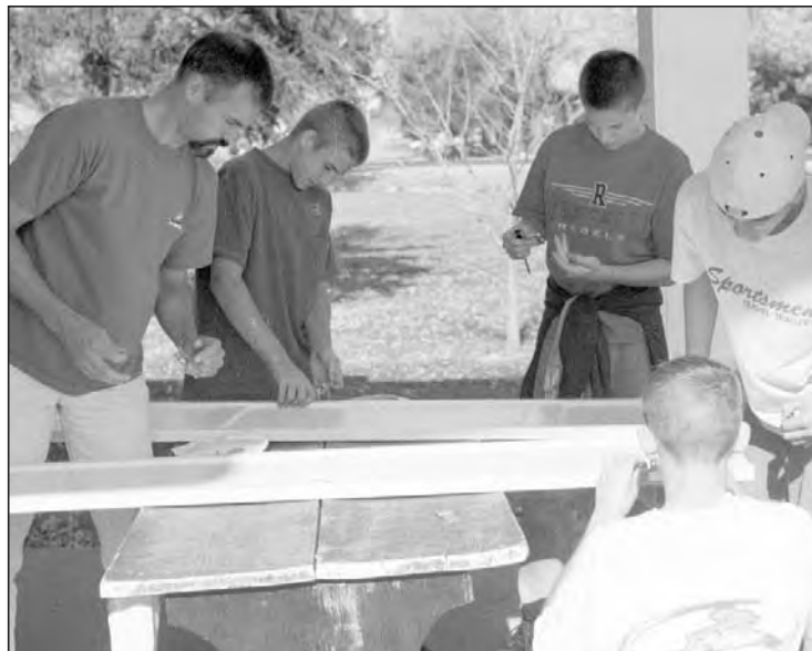
Pastoral council president Matt Braun (left) helps Nativity School students install new hinges on freshly painted doors during a recent service day. Later they reinstalled the doors in the parish office.
