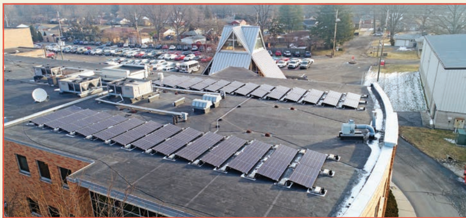
Recently installed solar panels sit on the roof of Cardinal Ritter Jr./Sr. High School in Indianapolis. In addition to reducing the school's carbon footprint and utility costs, the panels are being integrated into its science and theology lesson plans. (Submitted photo)
