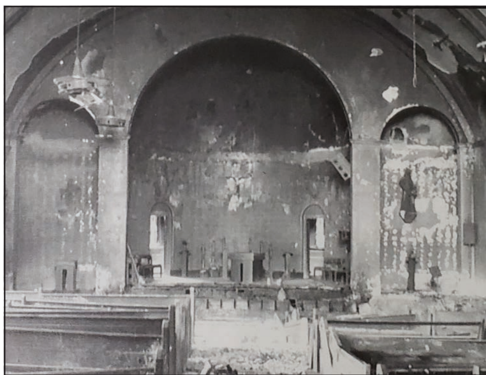
These photos show the extent of damage to the former St. Anne Church in New Castle due to an arson fire in 2007. (Photos courtesy of St. Anne and Her People by Doug Magers, Providence House Publishers, 2010)
